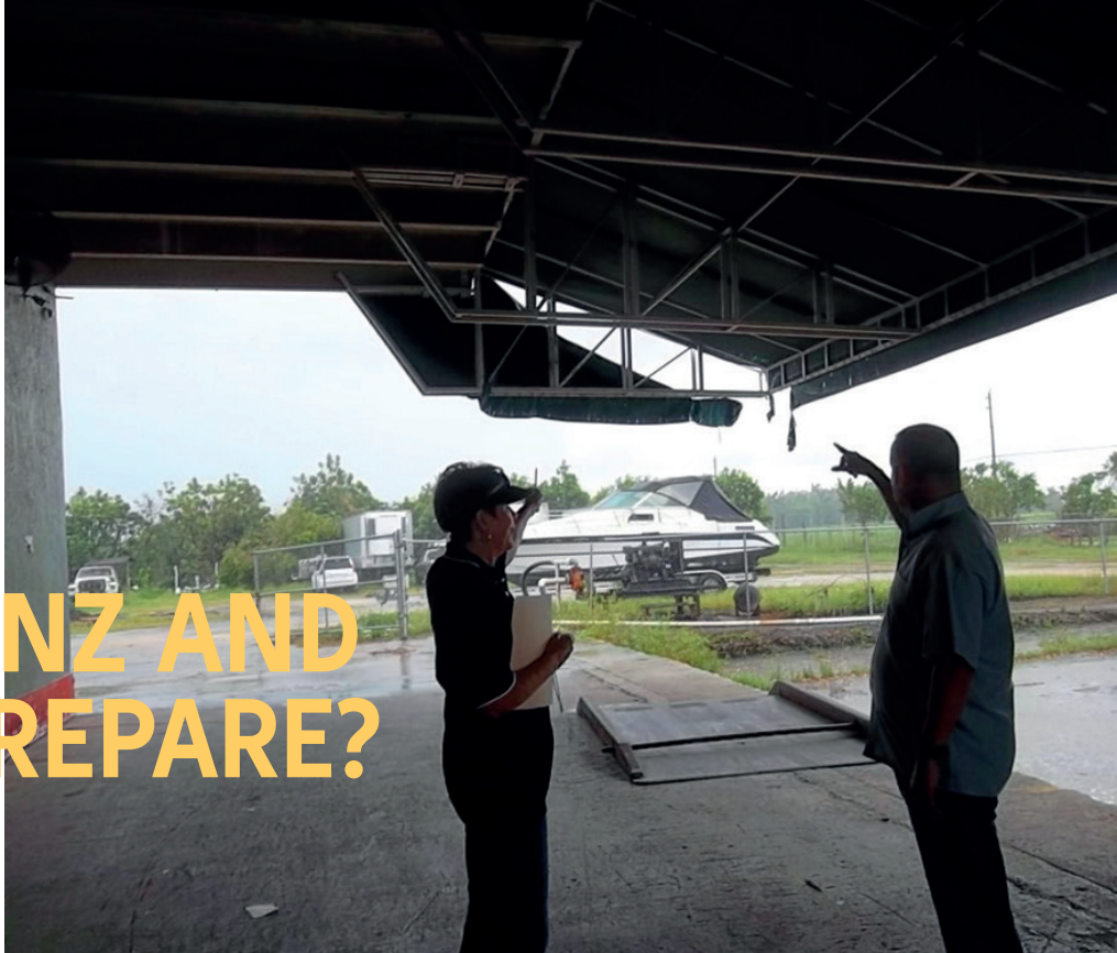
Allianz Claims Adjuster in Sebring, Florida inspects roof damage caused by Hurricane Irma Source: AGCS
