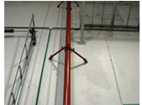
Sprinkler riser with sway bracing.
