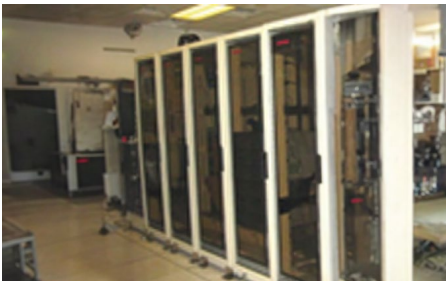
Computer server racks anchored to the floor.
