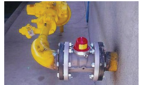
Seismic shutoff valve for natural gas line.
