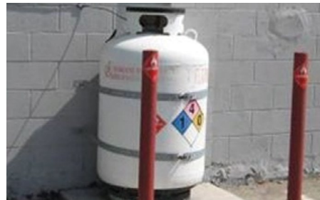
Flammable liquid tank strapped to wall.
