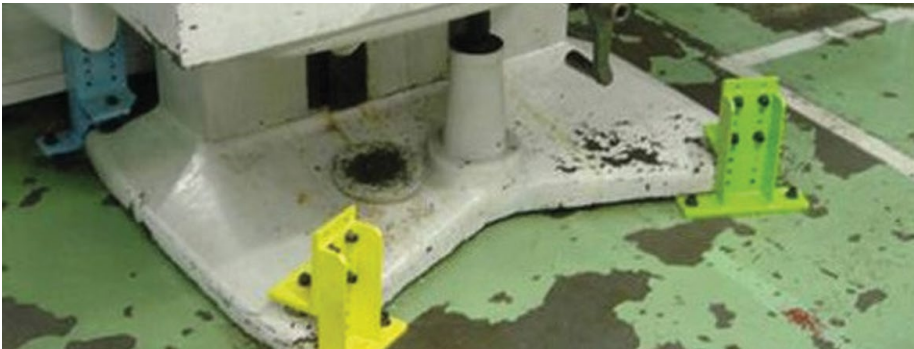
Production equipment anchored to the floor.
